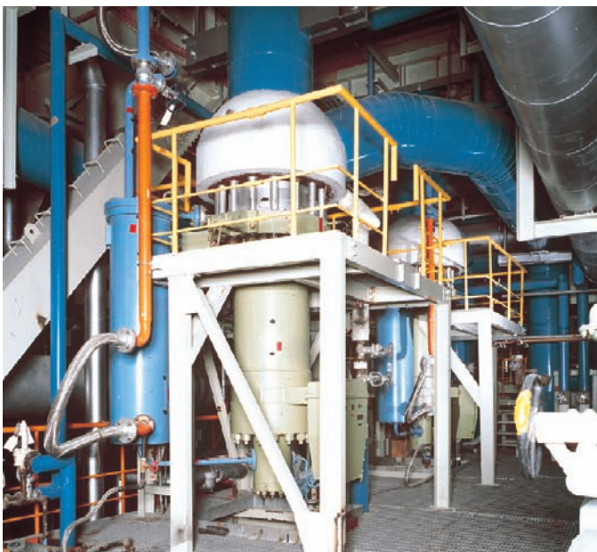
Hokkaido Electric Power Co.,Ltd. Tomatou Atsuma Power Plant 600MW, Japan
