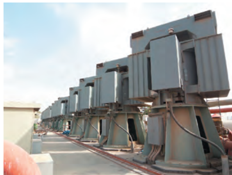
13 nos. of φ 1400 cooling water pump (PUBLIC AUTHORITY FOR INDUSTRY, KUWAIT)
