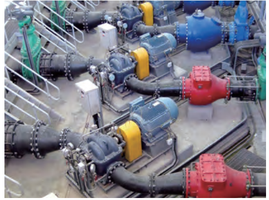
φ 400 Main pumps (OLD SALWA PUMPING STATION, QATAR)
