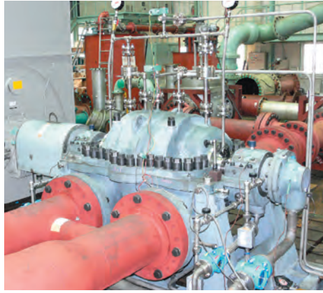
φ 300 Main pump (SHUQAIQ IWPP PHASE II, SAUDI ARABIA)
