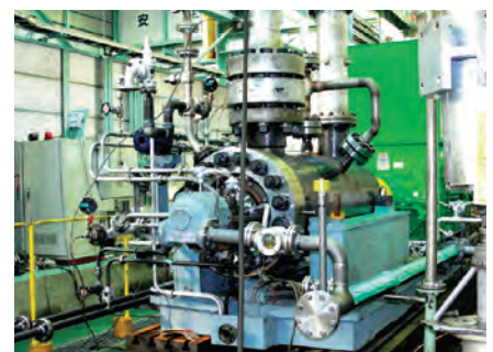
HP/IP Boiler feed pump (RATCHABURI POWER COMPANY LIMITED, THAILAND)
