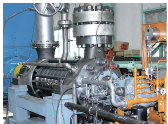
HP/IP feed water pump (E. ON UK ISLE OF GRAIN POWER STATION, UK)
