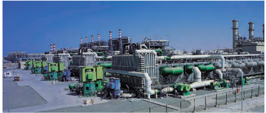
M.S.F. seawater desalination plant with various seawater pumps (AL TAWEELAH A2 DESALINATION PLANT, U.A.E.)
