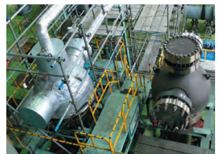
φ 300 Boiler circulation pump (NTPC KORBA POWER STATION, INDIA)
