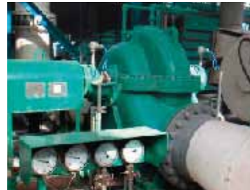
Closed cycle cooling water pump in power station
