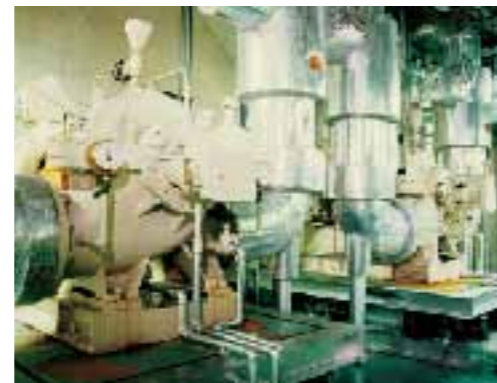
Cold water booster pumps in air conditioning equipment
