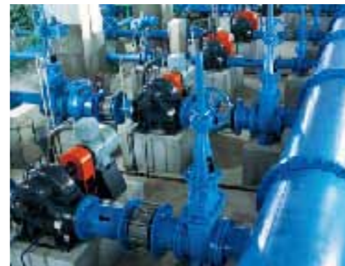
Distribution pumps in water works plant
