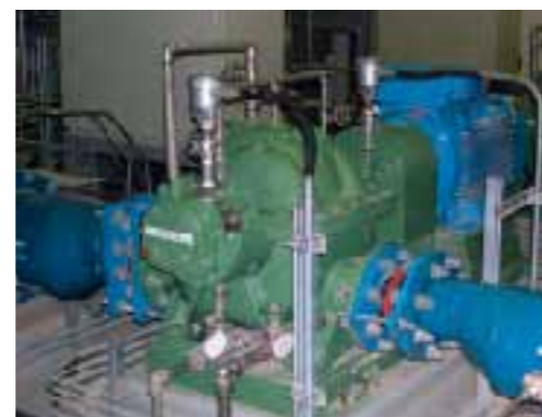
Potable water recirculation pump made of duplex stainless steel for water transmission scheme
