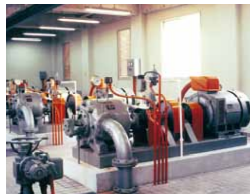
Distributing pumps in a small-capacity water works
