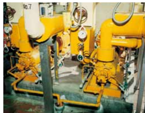
Boiler feed pumps in district heating and cooling plant
