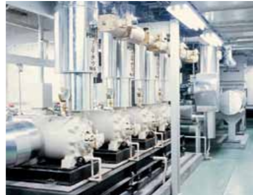
Booster pumps in building services application
