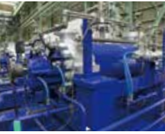
Boiler feed pumps for power plant in Argentina
