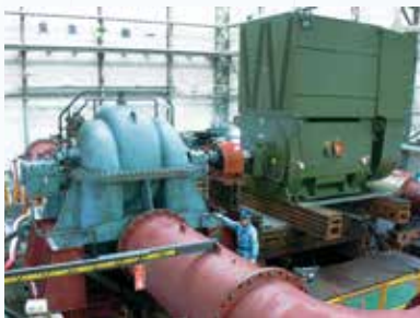
Cooling water pump for one of the largest ammonia plants in the world
