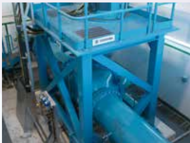
Reverse-rotated pump water turbine
